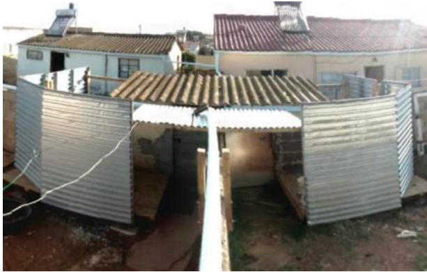
Water reticulation system - conversion of existing outhouses to accommodate Jojo tanks and solar PV powered filter and pumps.
